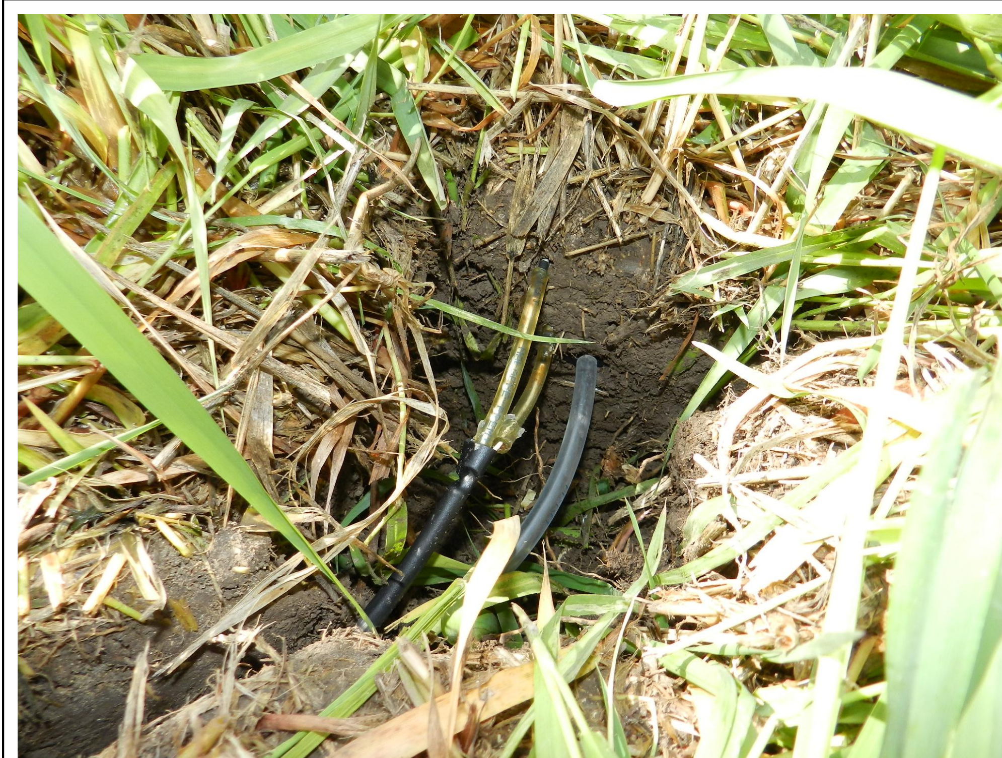
Figure 2. Installed soil sensors
